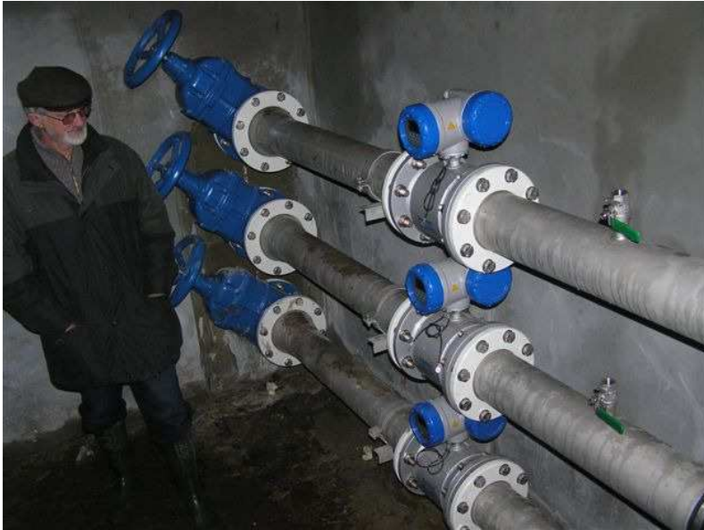
04.12.2007 – Piping, flow meters and valves in outflow structure
