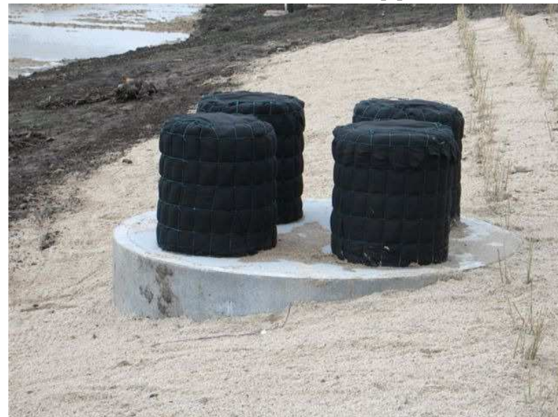
01.11.2007 Vertical sand filter
