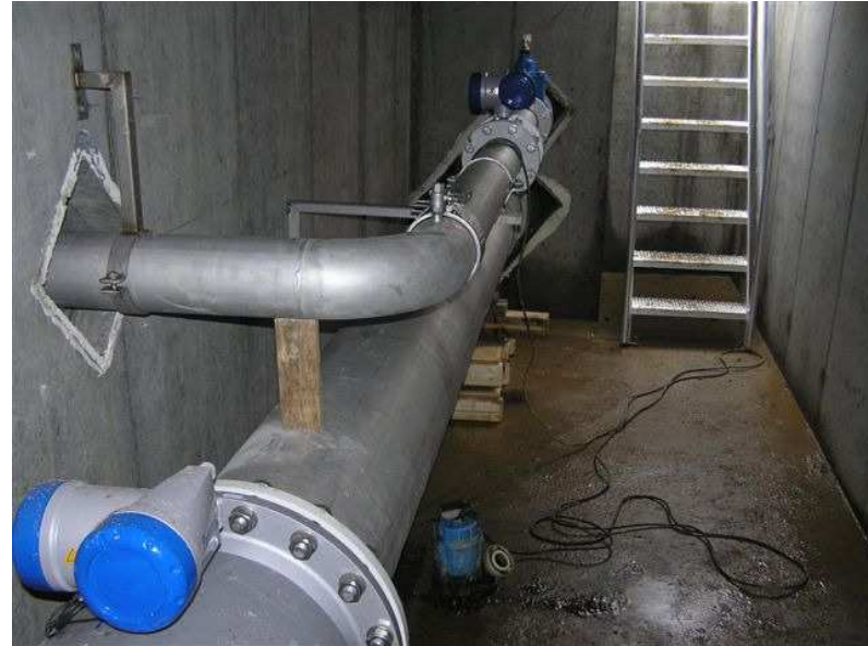
11.03.2008 – Piping and flow meters installed in inflow structure
