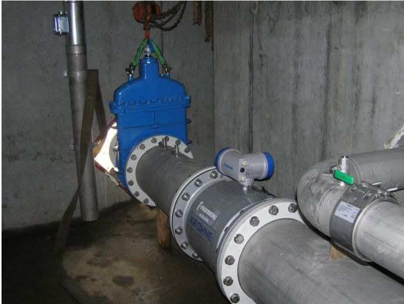
11.03.2008 – Piping, flow meter and valve in inflow structure
